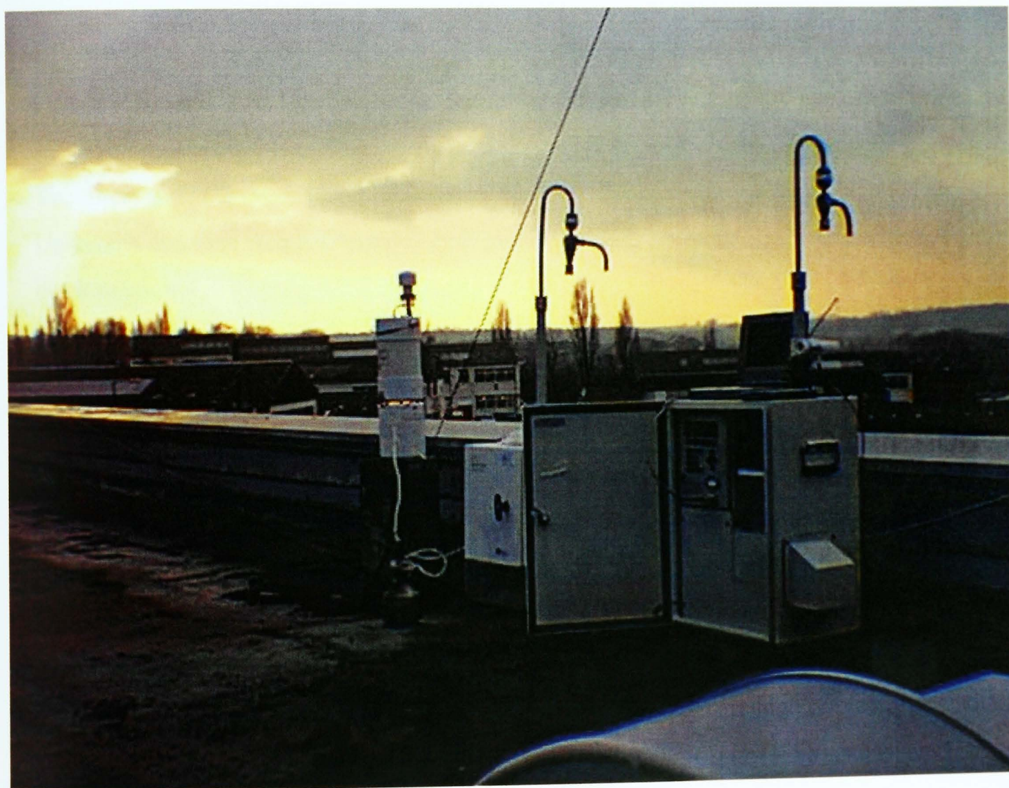
Figure 34: The Partisol 2000 and AirMetric sampling equipment on the roof at Middlesex University, North London, (information being downloaded from Partisol).
