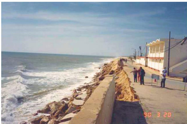
Figure 4. Destruction of the seawall and road in Praia de Faro caused by the impact of storms in 1990 (photo by J.A.Dias).
