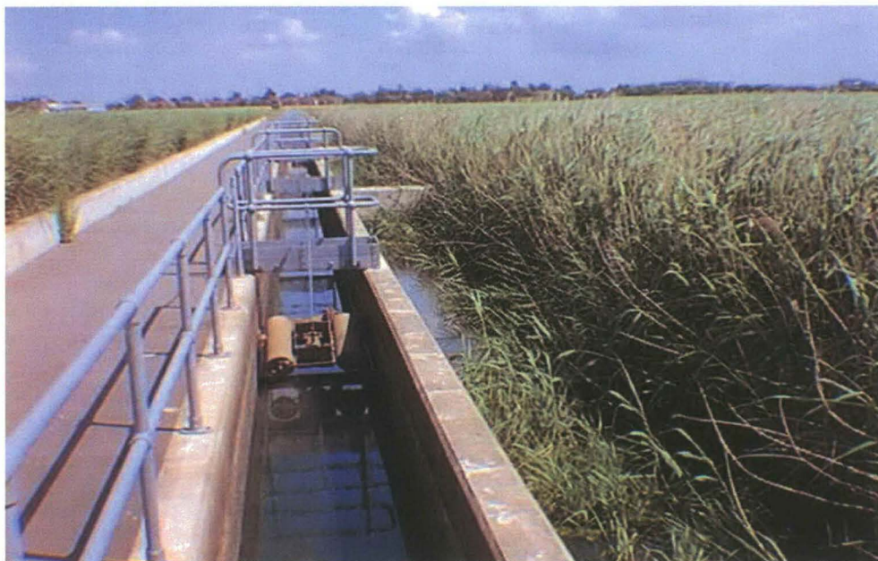
Figure 2.7 View along an exit channel for the sub-surface flow reedbed system showing the outlet flow control mechanisms
