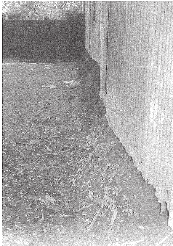
(b) Outside an MC house, outside wall decayed after 1988 flood (Tangail)
