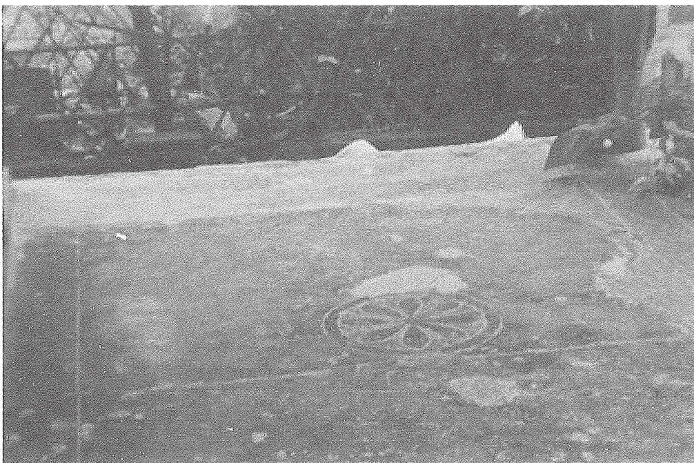
(b) A brick floor damaged subsequently after 1988 flood - not yet repaired
