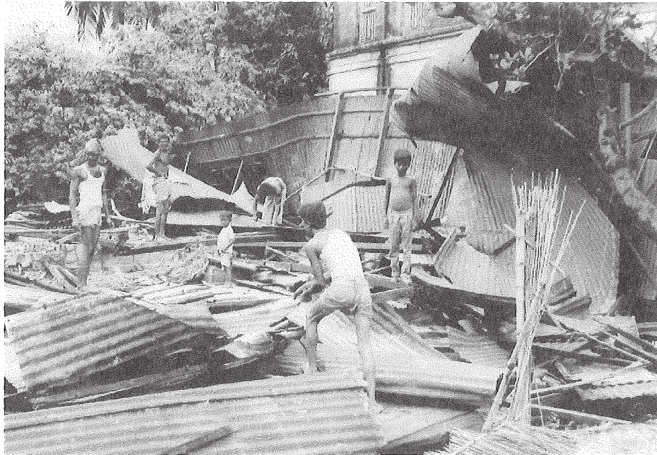
(a) Huge destruction to houses caused by tidal surge and cyclone (1991)
