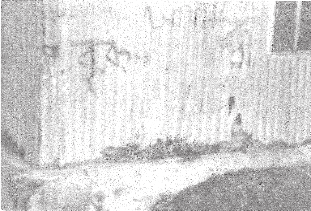
(a) A BC house with wall and floor decayed subsequently (1988 flood) - not yet repaired
