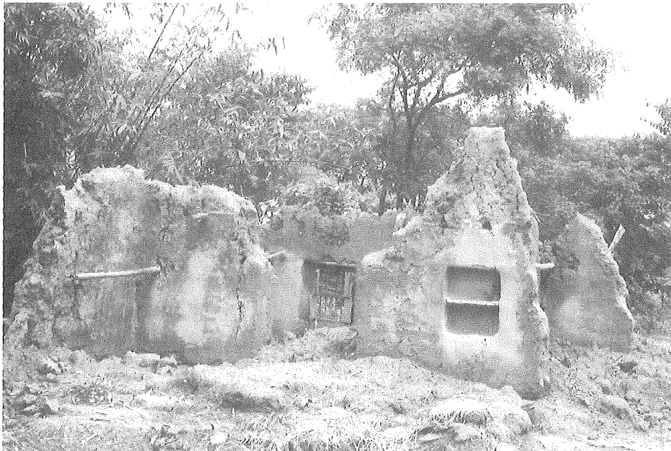
(a) An MM house completely destroyed by flood
