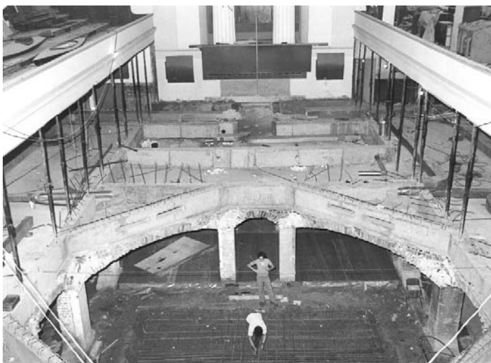
Image 82: No turning back: the first phase in the crypt and ground floor under construction
