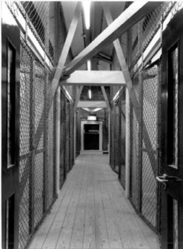
Image 86: Storage 'cages' in the roof that were a key to flexibility. They are now offices
