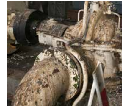
Decommissioned pumping apparatus
