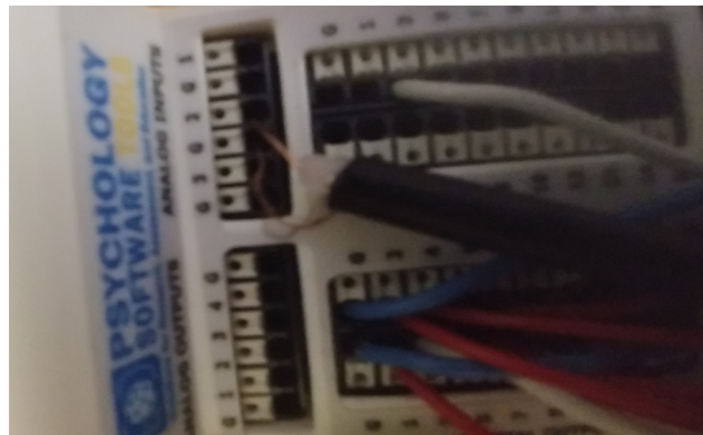
Figure 6. Wired Analog Input 2 of the Chronos expander. The BNC cable (black) was cut and unsheathed. The live cable was attached to Analog Input 2 and the ground wire was attached to the ground.
