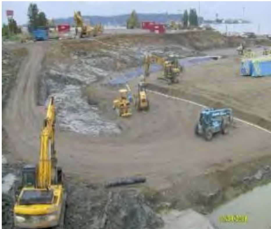
Figure A-7 Construction site in Blaine, WA, USA at the Canada/USA border.
