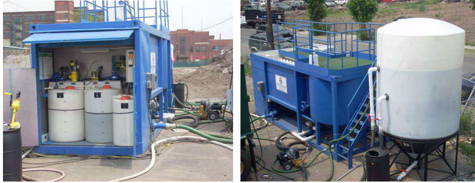
Figure 21 WetSep Filtration System in New Jersey, U.S.
