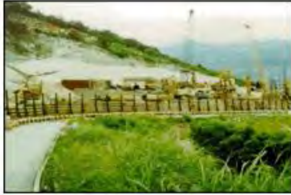
Figure A-1 Extensive site coverage of the slope stabilization project at Kau To.
