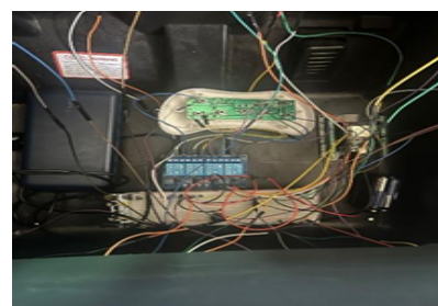
Figure 17. Hardware Components Mounted within the Platform
