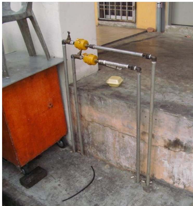
Photo 4.39. Unprotected waterlines in parking lot. No protective bollards to prevent cars from hitting them. Skudai.
