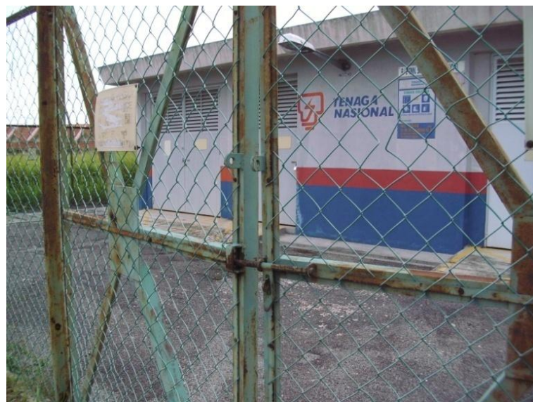
Photo 4.36. Unsecured electrical substation. Skudai.
