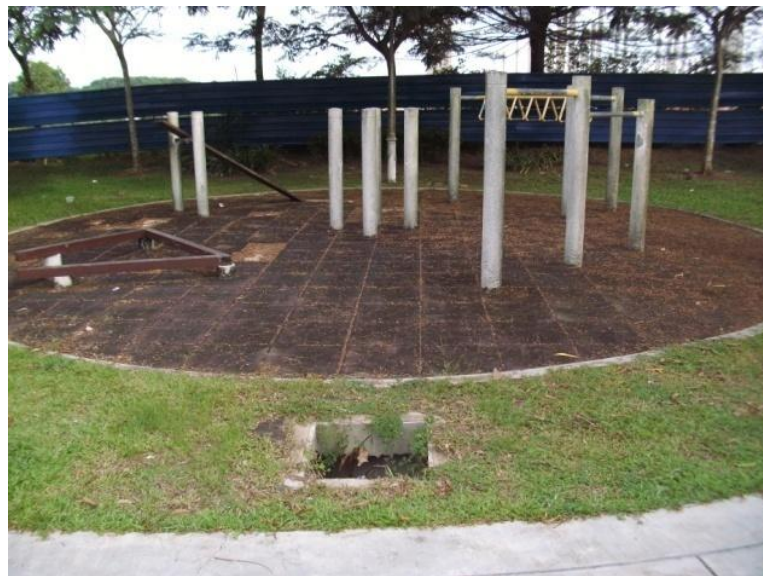
Photo 4.41. Open man hole near playground. Skudai.
