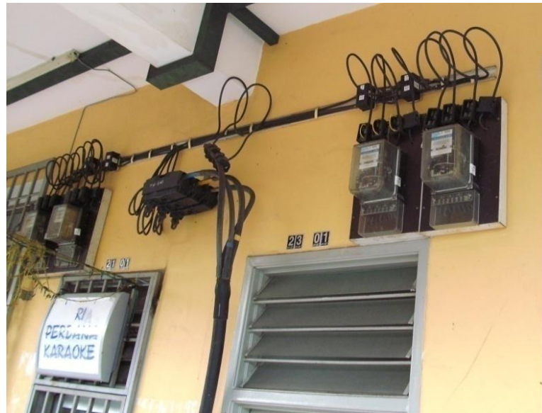
Photo 4.35. Power entrance to commercial buildings. Skudai.
