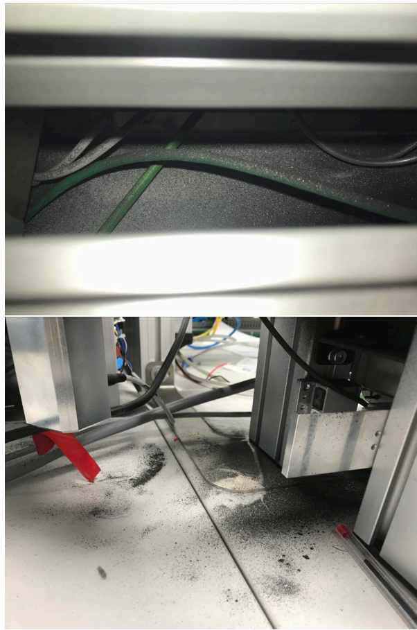
Figure 4.6: Aftermath from conveyor failure
