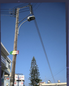
POLE H=5M WITH 70 W H.P. SODIUM
