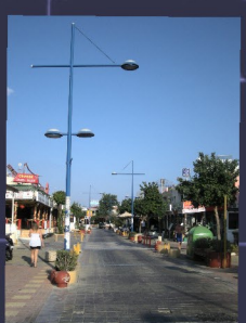
POLE H=5M WITH 70 W H.P. SODIUM LAMP+ HIT LAMP 150
