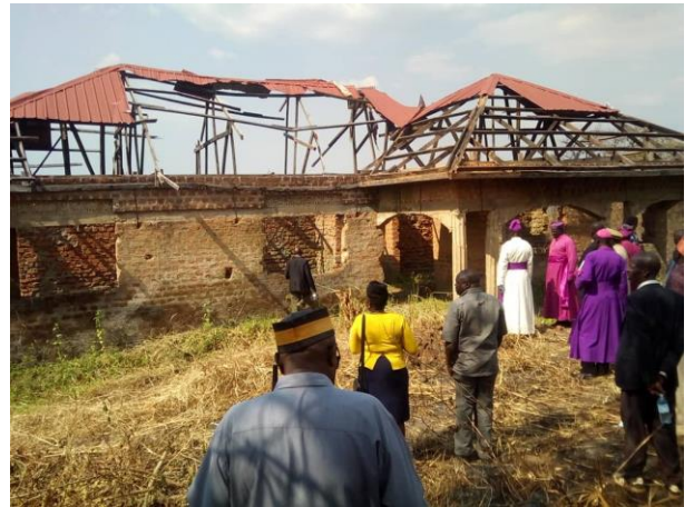
Photo 2 Church leaders plan to rebuild destroyed St. Joseph primary school: Photo by: Deco, June 2020
