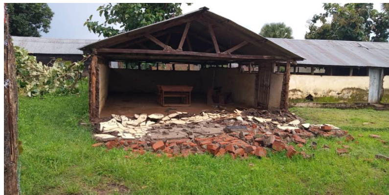
Photo 18 XXXX Govt primary school collapsed because of poor construction & absence of PTA supervision. Photo by: XXXX 27 th Sept 2022.
