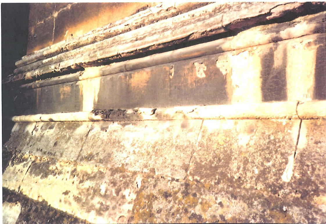
Plate 2.2 Photograph Showing Black and White Crusts at Lincoln Cathedral.
