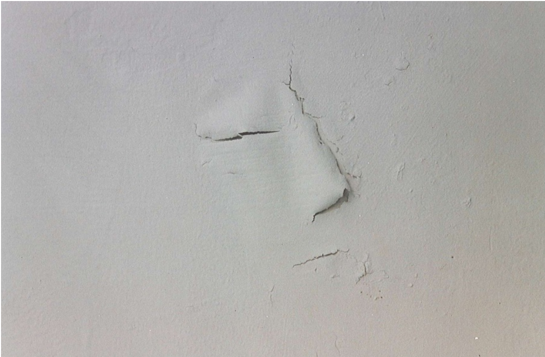
Figure 3: Shaun Martin, The ready-made self portrait 2000 – 2005. Original lost. Peeling wall plaster.
