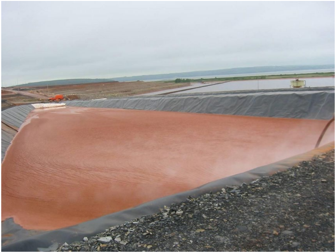
Figure 64 Demonstration Cell filling in 2007
