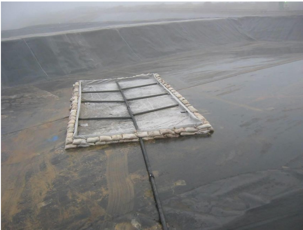
Figure 48 Seepage collection tray in floor of cell 2006
